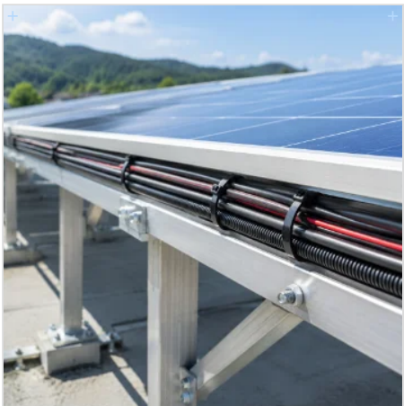
Solar and outdoor installation
